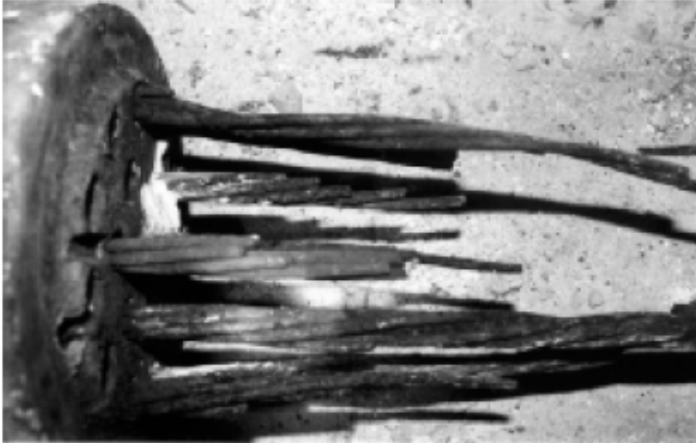
Figure 1. Failed Tendon at Niles Channel Bridge [4]
