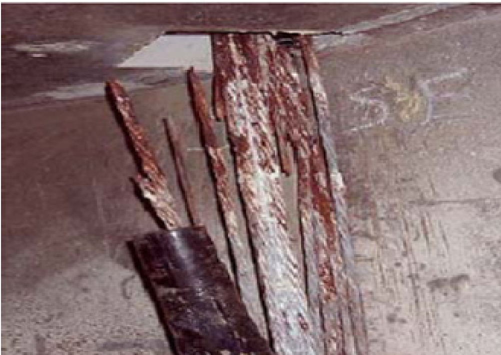
Figure 2. Failed Tendon at Sunshine Skyway Bridge [5]
